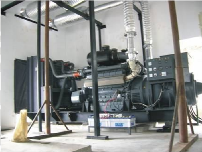
Engine Installed On Site
